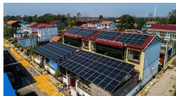
The residential photovoltaic power generation project supported by the Bank in Lankao County.
