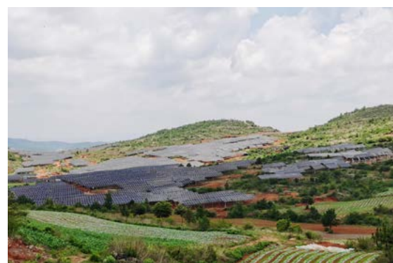
Yunnan Branch supported project of Zhanyi Lingjiao agricultural photovoltaic power generation.
